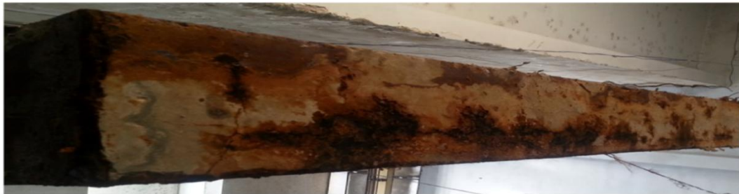
Fig.21. Deterioration of the concrete against corroded rebar for sample
